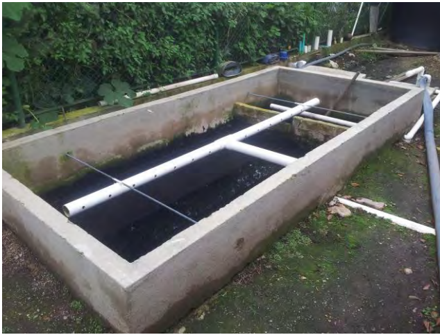
Figure 26: Sludge drying zone
